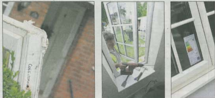
Out with the old and in with the new: Workmen replace the old wooden windows with PVC-U.
